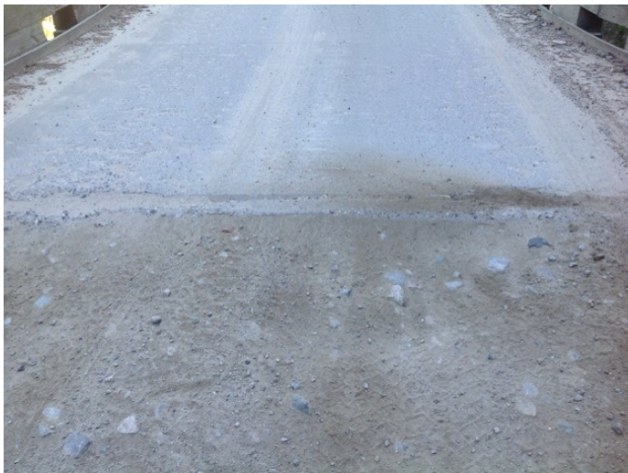
ballast wall and deck damage on both approaches
