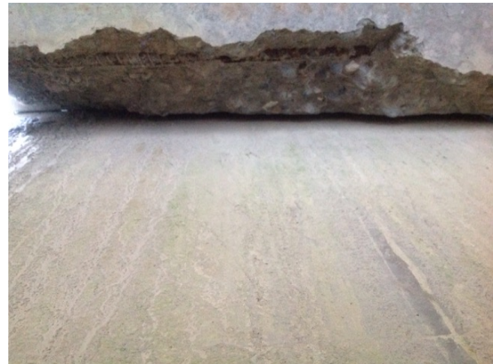
panel damage under left approach
