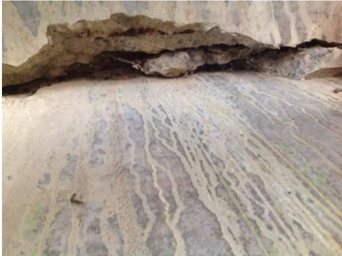
panel damage under right approach
